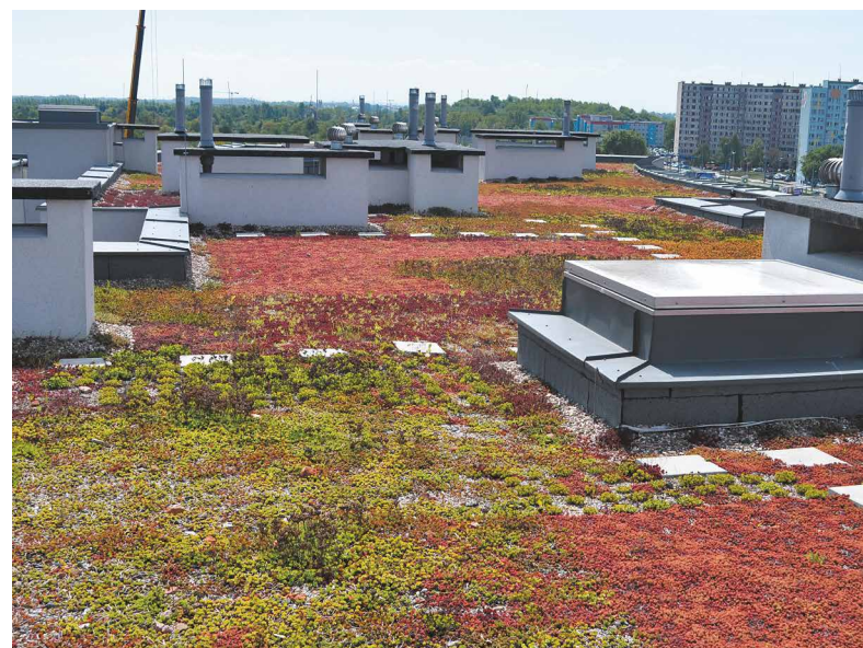
Sedum roof on a multi-apartment building in Wrocław, Poland / Photo: Marta Weber-Siwirska
